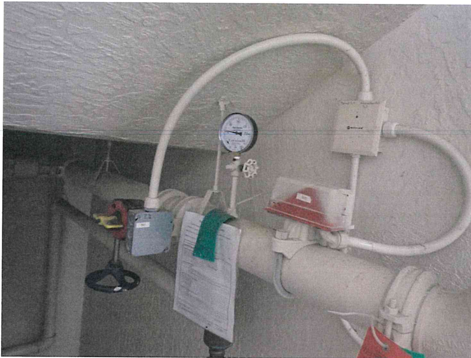
7. View of the fire suppression system.
