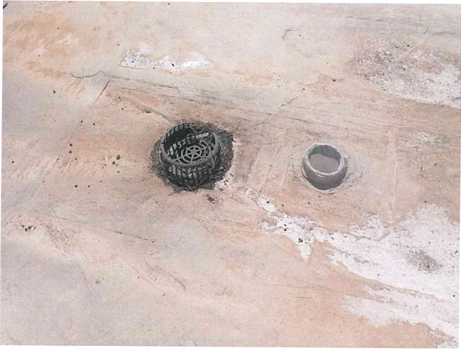
11. View of a roof drain and vent pipe on the flat portion of the roof.
