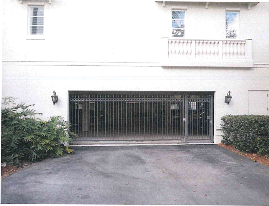
3. View of the parking garage entrance located at the northeast end of the building.
