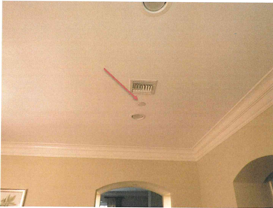
17. View of the typical recessed sprinkler head in the interior of the units.
