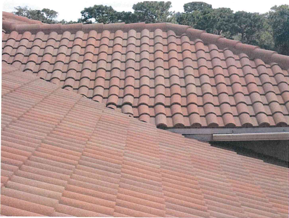
13. View of the loose/dislodged roof tiles on the northeast end of the building.
