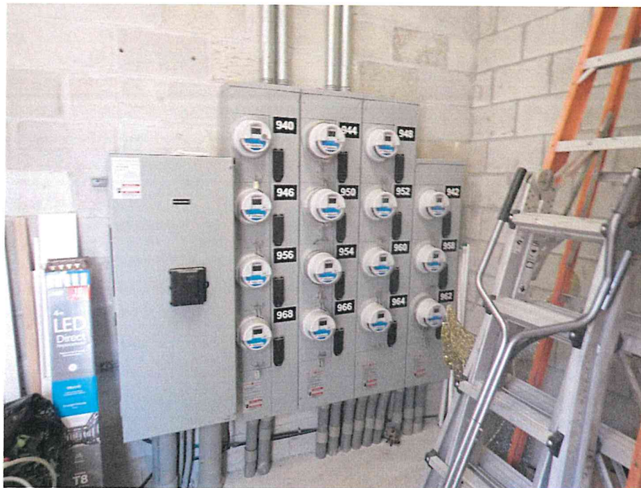
8. View of the electrical room.
